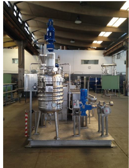
Bio-polymer production skid
