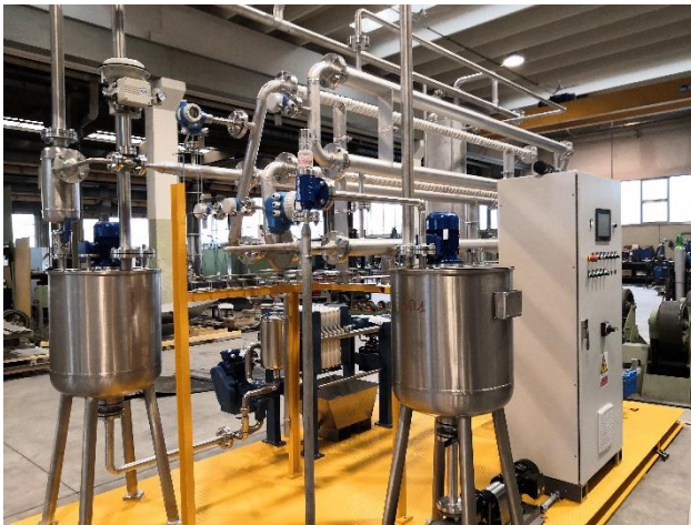
Hydro Thermal Carbonization pilot plant on skid
